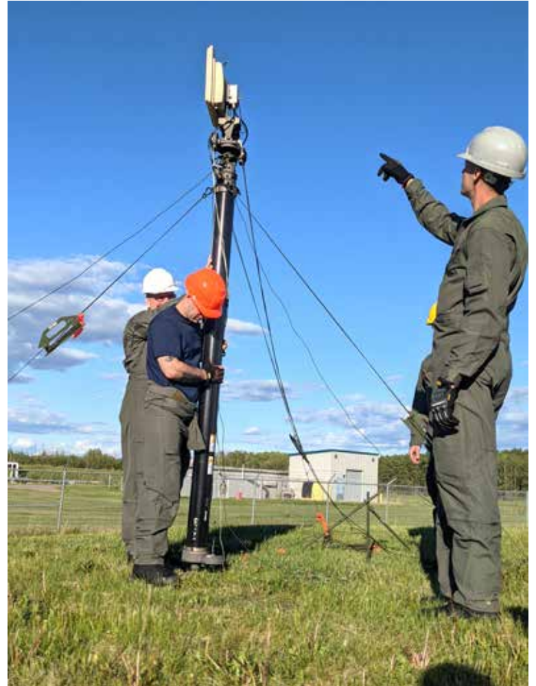
Members of the Maine Air National Guard’s 265th Combat Communications Squadron install communications equipment in support of Exercise Amalgam Dart at Canadian Forces Base Cold Lake in Alberta on June 12. PHOTO BY MAJ. BRENDEN WESTIN, MAINE NATIONAL GUARD
