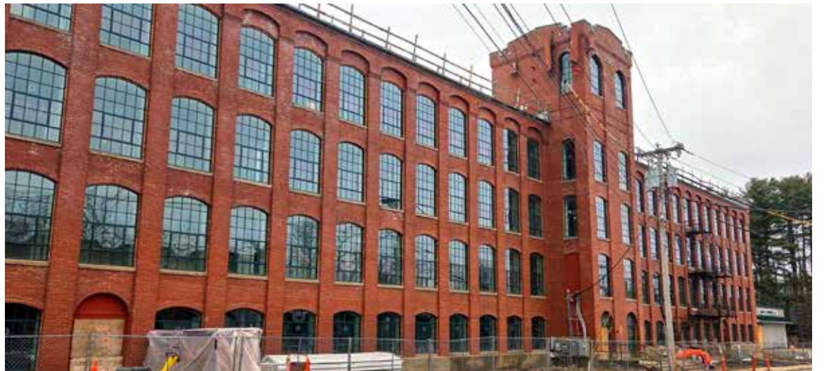
Jagger Mill in Sanford is currently under renovation. PHOTOS BY THE SANFORD REGIONAL ECONOMIC GROWTH COUNCIL
